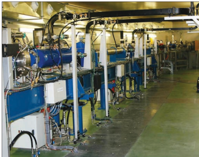
ALBA's 100 MeV linac works at 3 GHz with a 3 Hz repetition rate.
